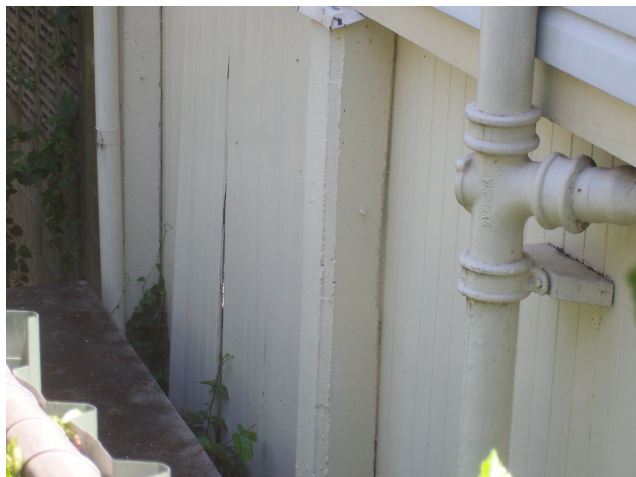
Rotten and deformed timber of asbestos ridden derelict hovel.
