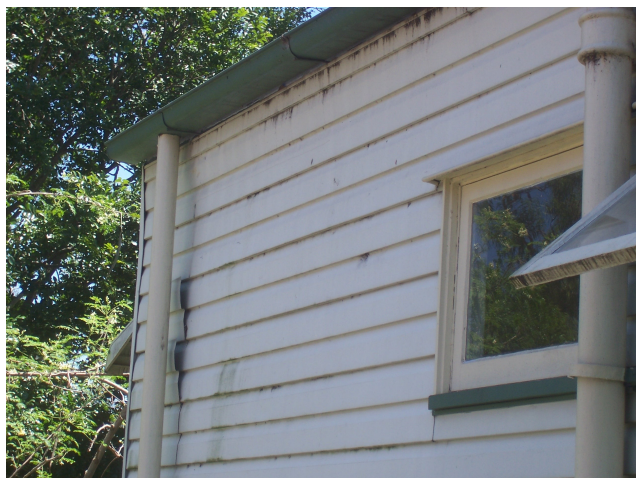
Loose cladding on hovel as there is nothing substantial beneath to which cladding can be secured.
