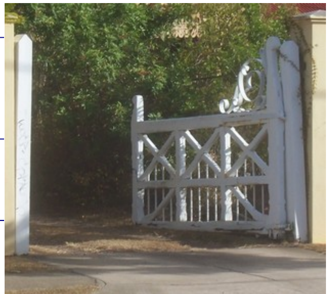
Derelict gate at far end of front fence of 41 Gray Road. Not much movement there for a while.
